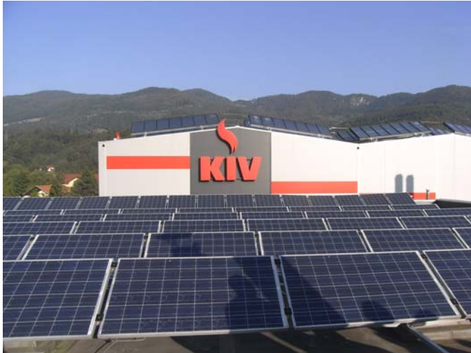
Energetika Vransko PV plant and solar thermal installation on KIV
