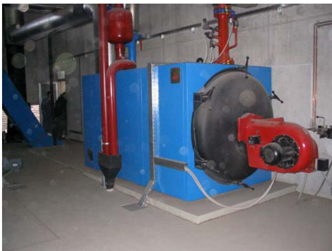
Smaller of the two KIV biomass boilers at Energetika Vransko district heating
